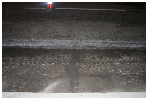
Cracking to the existing road surface
