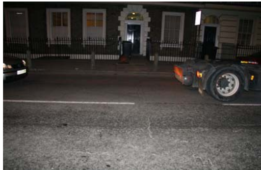
Cracking to the existing road surface
