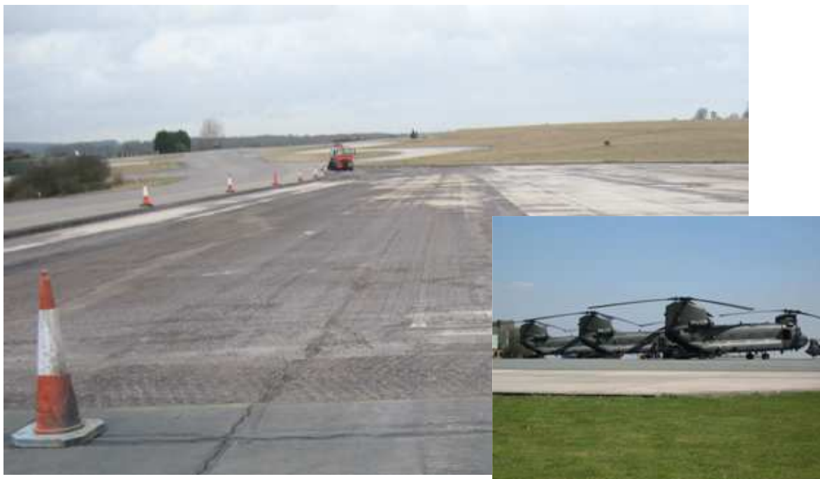
Centre: Overlay milled-off ready for Glasstex installation. Right: Repaired airfield for Chinook helicopters
