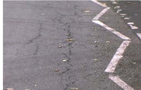
Cracked asphalt before the repair
