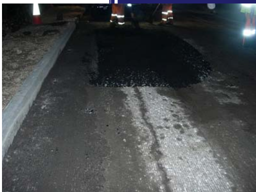
View of the planed/damaged surface
